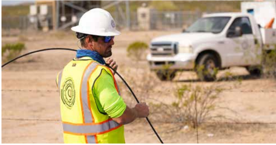
Fiber Technician conducts work out in the field. Photo Courtesy of Gila River Telecommunications
